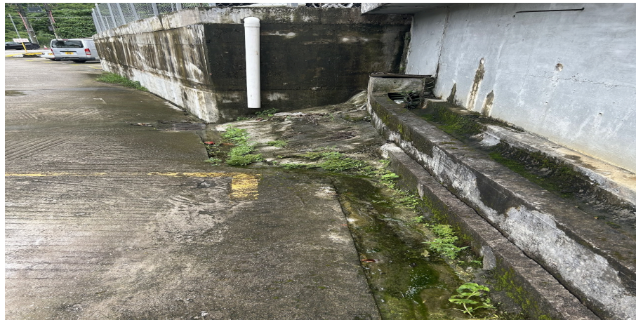
Figure 25: On site drain
